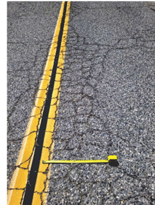
Photo 3 closeup of road surface showing alligator cracking, longitudinal cracking, and weathering.
