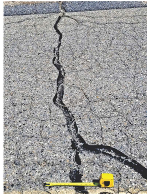
Photo 2, closeup of road surface, showing patched and reopened transverse cracking, alligator cracking, edge cracking, weathering, and locally polished aggregate.
