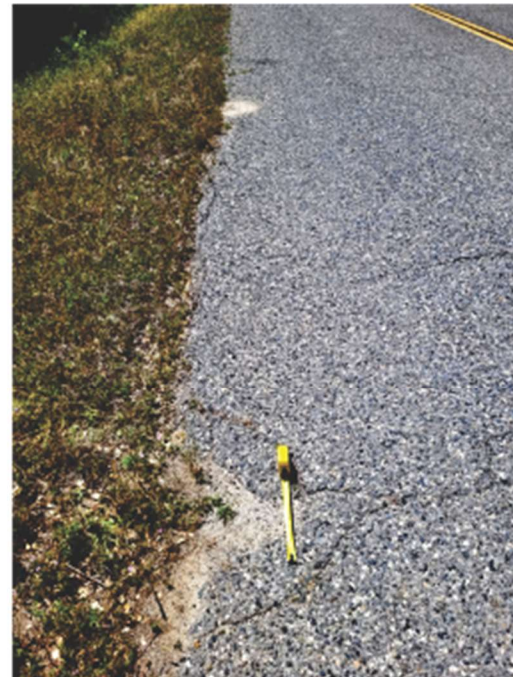
Photo 2, closeup of road surface, showing edge cracking along east side of road, transverse cracking, and weathering.
