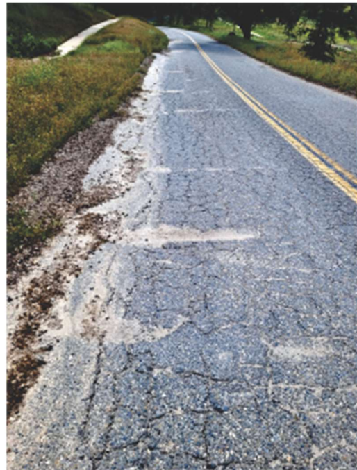
Photo 1 looking east along north edge of road surface showing alligator cracking, edge cracking, longitudinal/transverse cracking, and weathering/ravelling of road surface.
