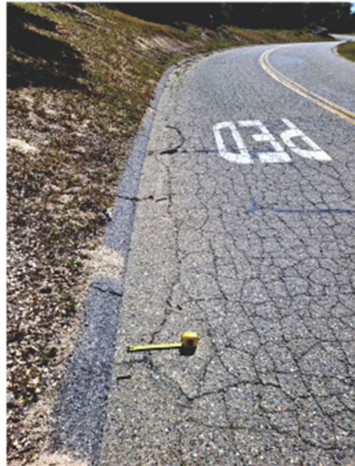
Photo 1 along northeast side of road looking southeast showing edge cracking, alligator cracking, transverse cracking, cracking in HMA soil dike, and weathering of road surface.
