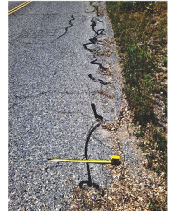
Photo 4 closeup of road surface showing patched edge cracking along west side of road, alligator cracking, longitudinal cracking, and weathering.
