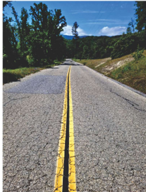
Photo 1 looking southeast showing alligator cracking, patching, and weathering of road surface.
