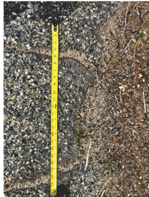
Photo 2, closeup of road surface, showing edge cracking and weathering.
