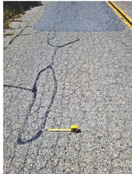
Photo 2, closeup of road surface, showing patched and reopened longitudinal cracking, alligator cracking, weathering, and locally polished aggregate.
