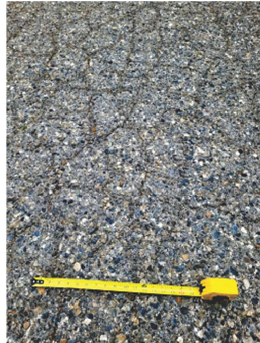
Photo 2, closeup of road surface, showing alligator cracking and weathering. Locally, exposed aggregate is polished but still angular.
