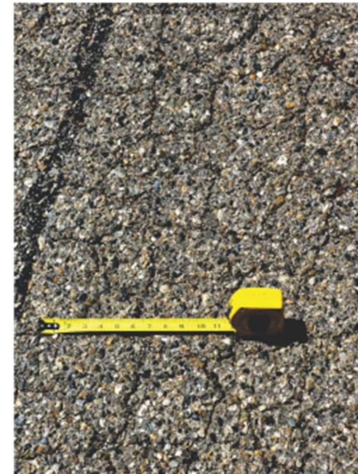
Photo 3 closeup of road surface showing alligator cracking, polished aggregate, and weathering.
