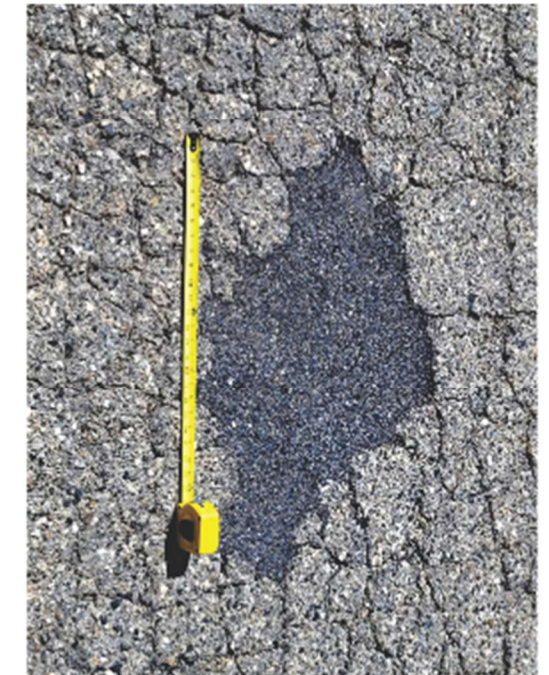
Photo 4, closeup of road surface showing alligator cracking, patched pothole, and weathering/raveling.
