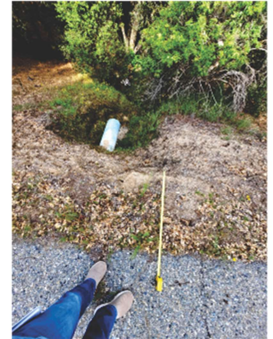
Photo 4 looking west along west edge of road showing erosion, possible piping, and loss of ground of road fill at buried storm drain outlet. Headscarp of the erosion scar approaches to within ~3' of road surface.
