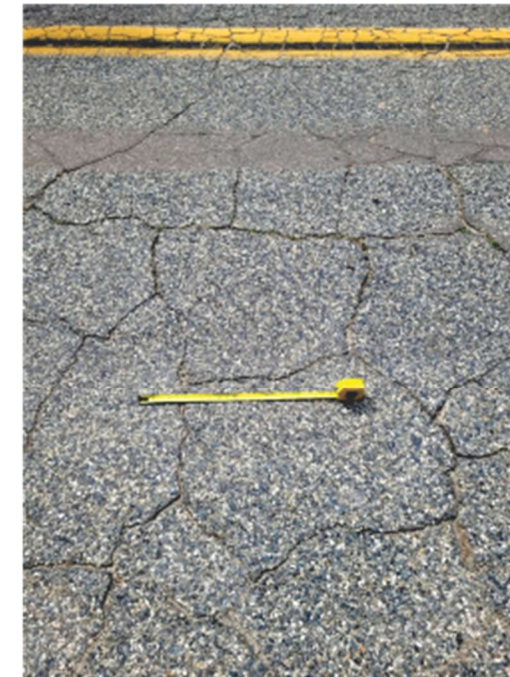
Photo 3 closeup of road surface showing block cracking, alligator cracking, depression, and weathering.
